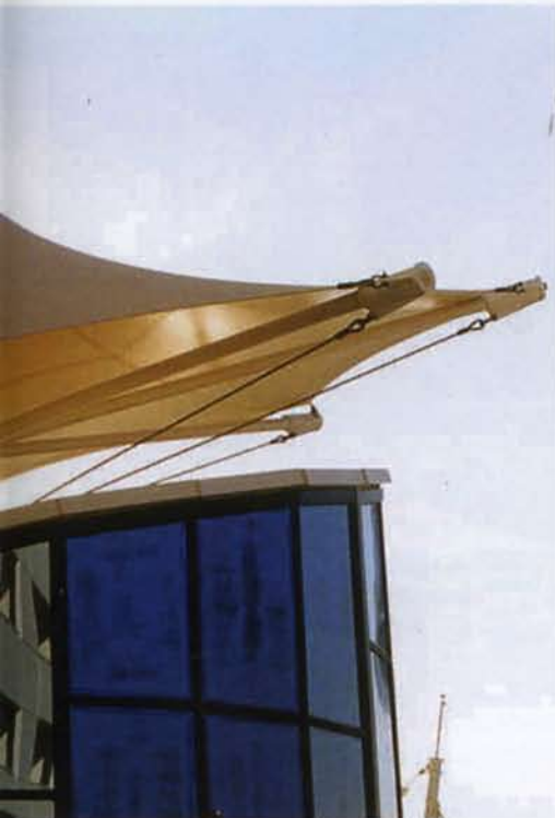
A threaded adjusting device elongates the catenary cables and provides tension for the canopy.
